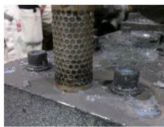
Figure 3 - Wire mesh filter pulled out of system for replacement.
